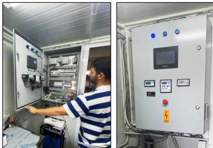
Figure 79 Photos of the control unit
