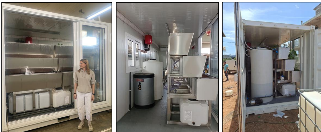
Figure 64 External and internal views of the vertECO® water treatment system installed vertically stacked modules with each module having a length of 1500 mm and a width tapering from 500 mm at the top to 400 mm at the bottom (Figure 64). This design facilitates even water distribution and creates a combined treatment volume of almost 1.8 m 3 .
