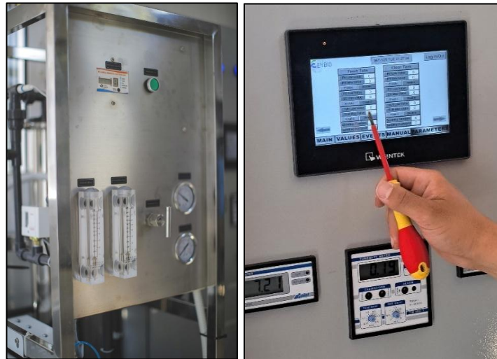
Figure 63 Reverse Osmosis Unit (left), Control Panel Display (right)
