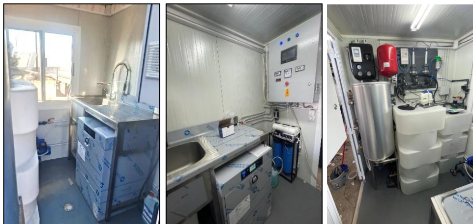
Figure 76 The DW unit (left), the basin (middle), and integrated water tanks for GRETA™ (right)
